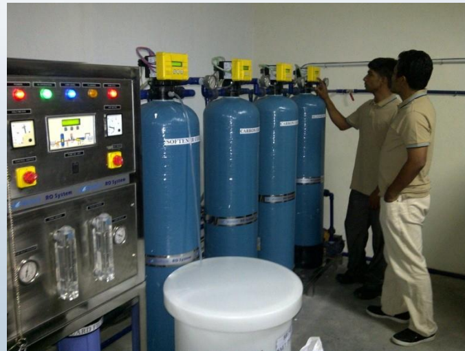
Reverse Osmosis Installation
